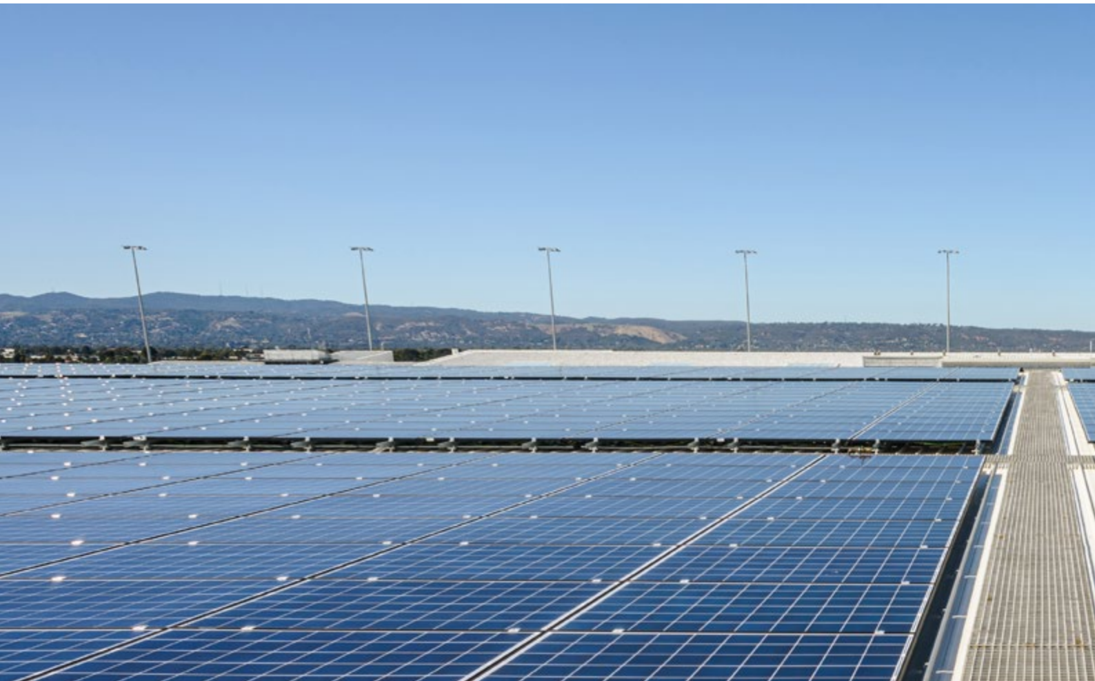
Figure 11-1: Installed Solar Photovoltaics on Multi-Storey Car Park Roof
